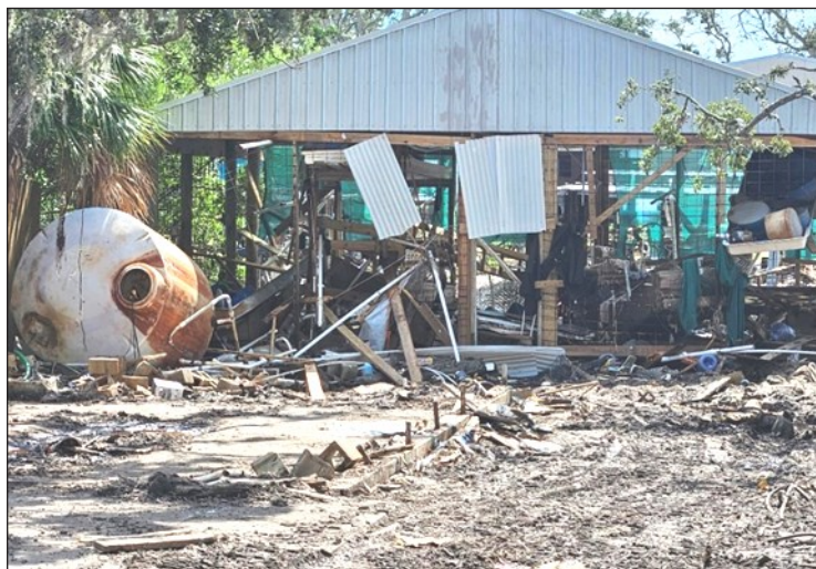
Clam hatchery in Cedar Key destroyed by Hurricane Helene. Photo credit: Leslie Sturmer
